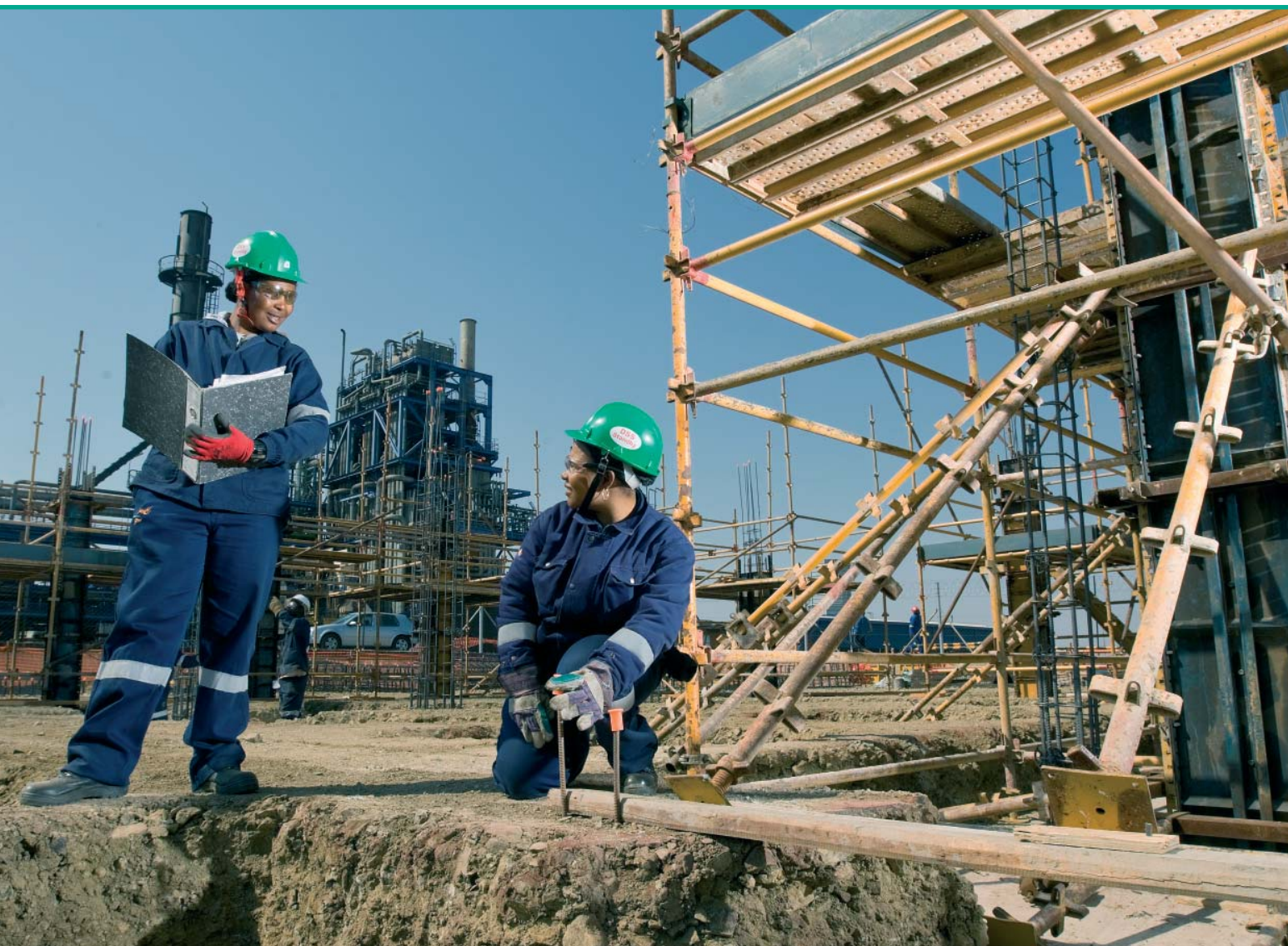
Safety standby contractors, Jerita Mokoena and Nomsa Radebe, check the construction site of the new Sasol Wax plant at Sasolburg for potential hazards.
