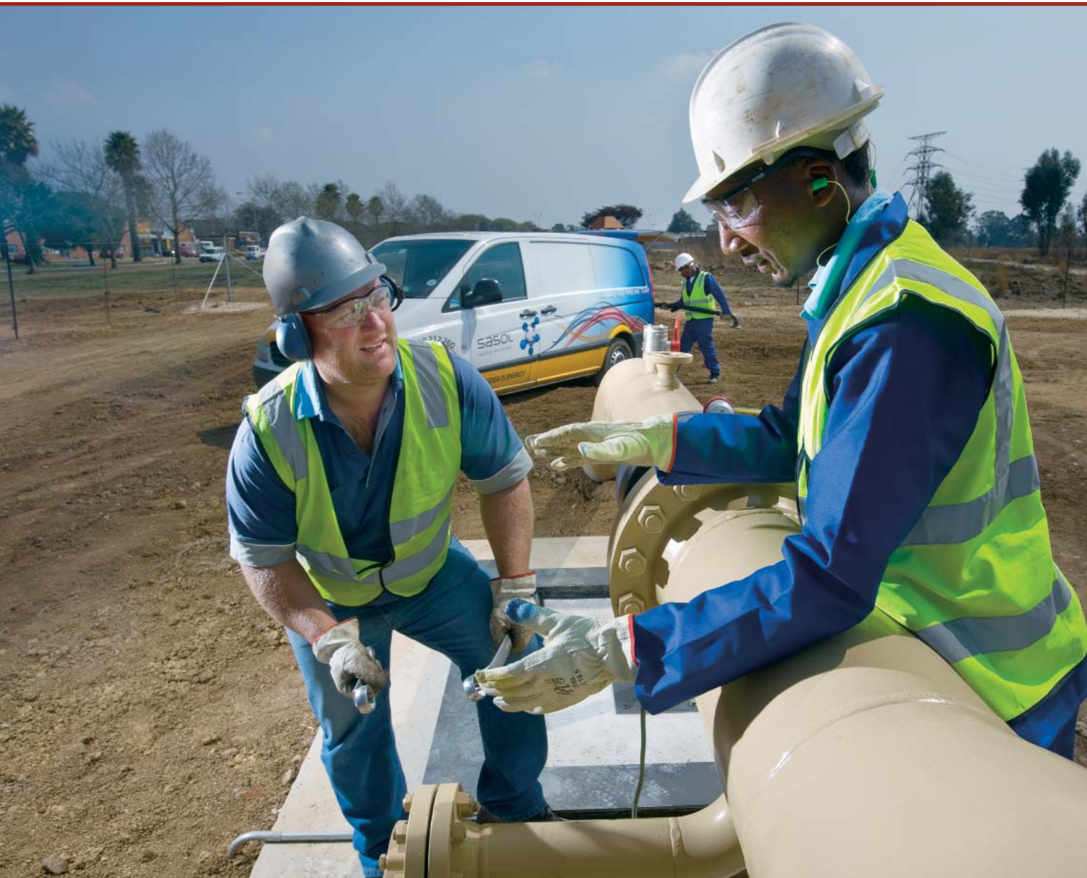
Sasol Gas continues to improve its safety performance and pipeline integrity. Christi Kapp and John Tabi conduct a maintenance inspection of the Springs Olifants gas pipeline.
