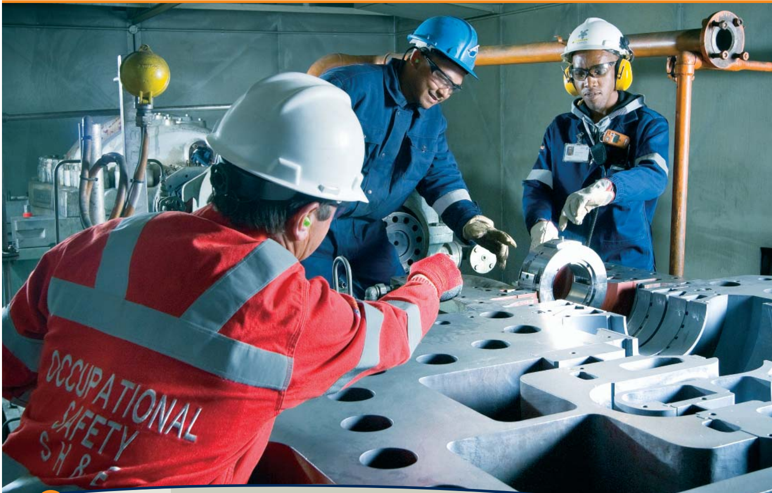
Dean Strijdom, Emile Slabbert and Lucius Gina engaged in the maintenance of a turbine compressor at the oxygen west unit at Secunda.
